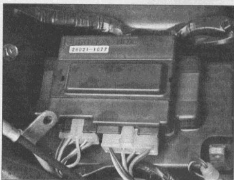
5.2a Most of the EN500 fuses, including the spares, are located on the junction box
